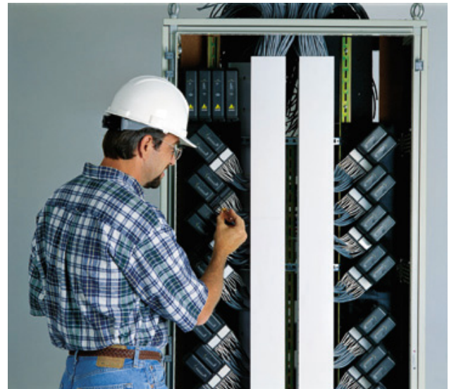
Vertical-mount I/O carriers mounted in a standard-sized cabinet.
